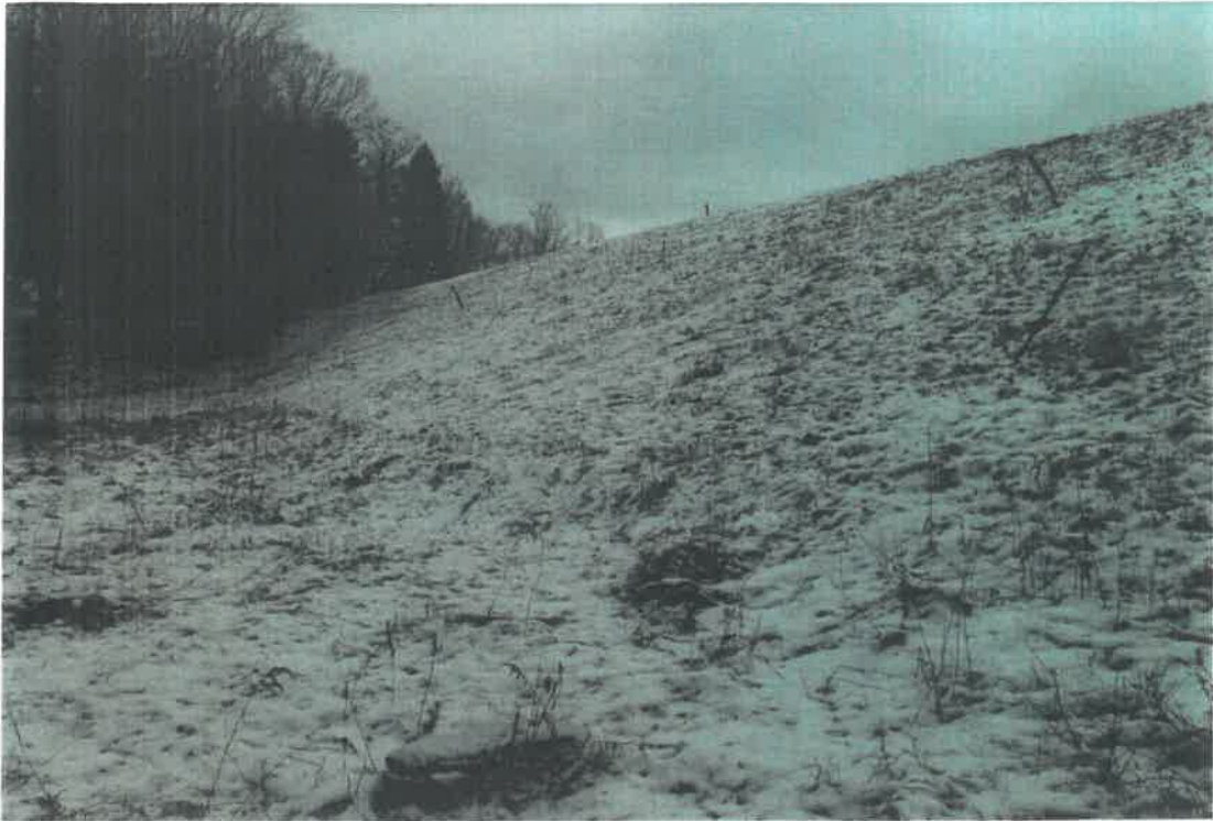
Photo 13 Dam ID# 243-1430 Martin Dunham Reservoir Dam 01/05/2024 Right downstream face of the dam
