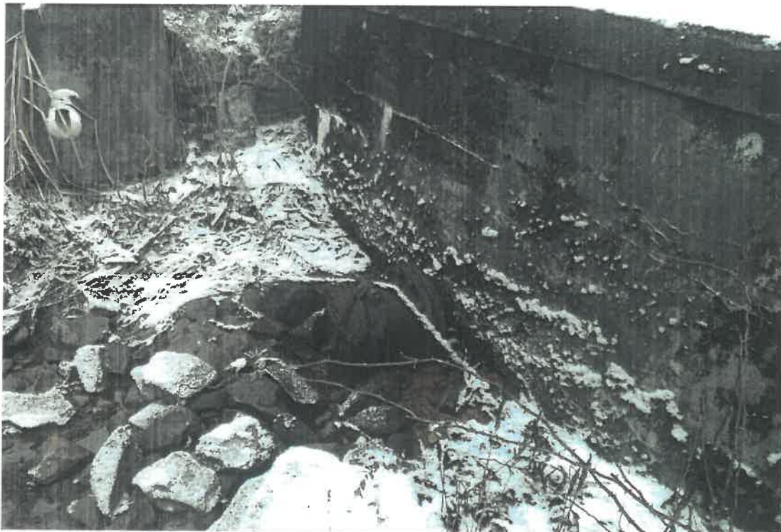
Photo 4 Dam ID# 243-1430 Martin Dunham Reservoir Dam 01/05/2024 Right (auxiliary) low level drain and toe drain
